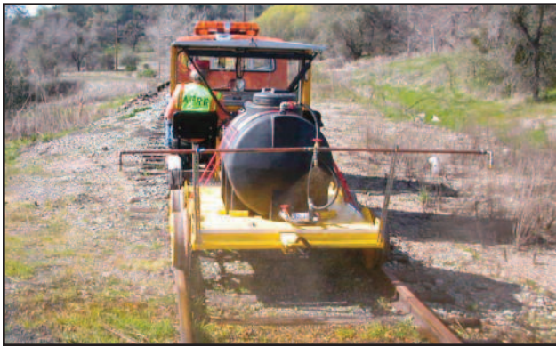
Photo by Larry Bowler RRCHS work crew spraying the Amadore Central right of way using "007" built by Grant Vogel.
