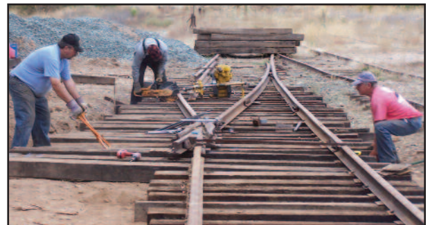
Photo by Robert Piacentini Greg Ockander, Joe Nemmer, and John Atkinson installing the first switch.
