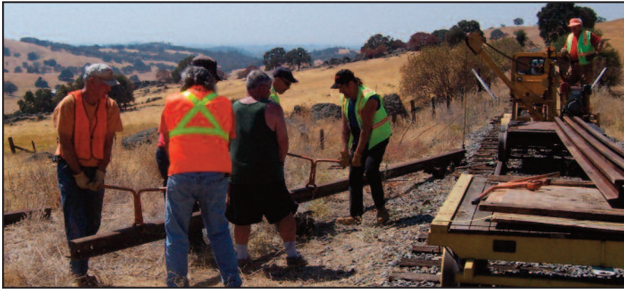
Photo by Robert Piacentini RRCHS work crew recovering rail from along the right of way for use in rebuilding the wye in Ione, CA.
